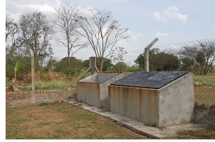
Figure 5. Two chambers in the burial area of the WWTP, for additional drying of the solids which is noted to be too humid. Source: (Y. Geber 2019).
