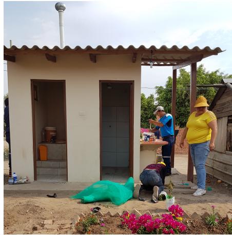
Figure 3. UDDT with grey water garden in Montero under construction by COSMOL. Source: (Y. Geber 2019).
