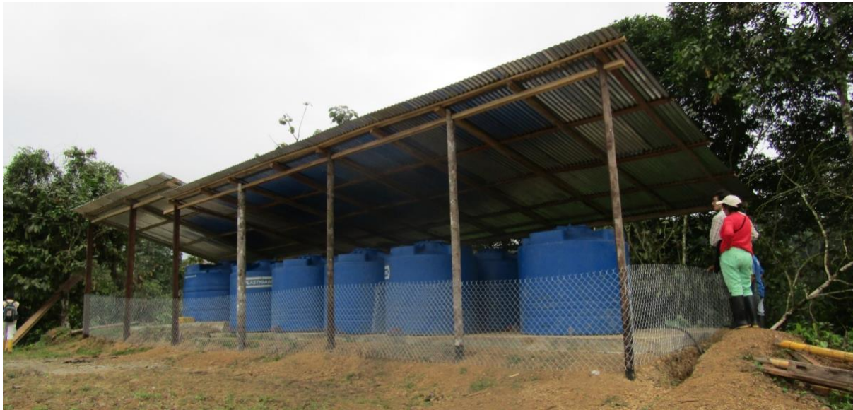
Figure 2 The treatment system tanks in San Salvador (December 2016).
