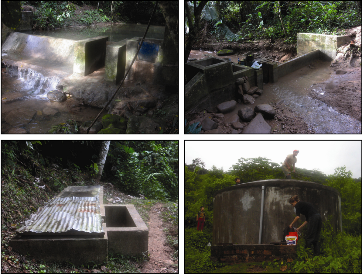
Figure 10 Parts of the water distribution system: point of capture (upper left) and the dam when emptied for cleaning (upper right), sand trap (lower left) and reservoir (lower right).
