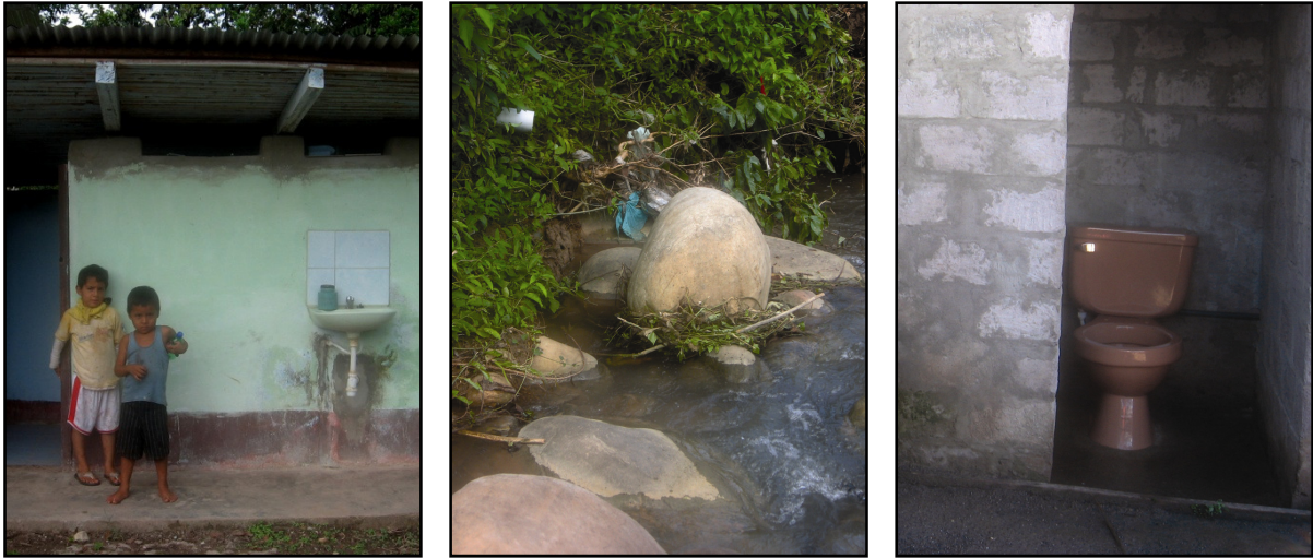
Figure 11 Blackwater systems in Nueva Vida. Toilet at the health center (left), wastewater discharge by the health center (middle) and one of the two household installations in use at the time of the study (right).
