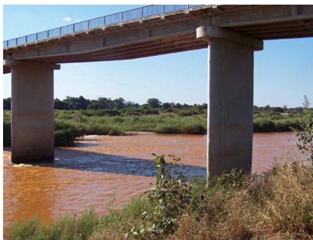
Figure 6.13. The EN1 road passing over at the EFR site. At the bridge pier closest in view is a water measurement scale (Photo Lovisa Lagerblad).
