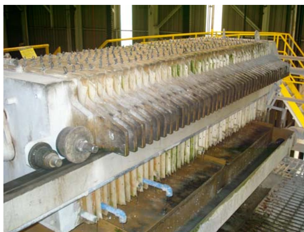
Figure 15. Filter press for dewatering of sludge.
