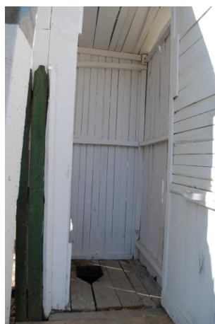
Figure 32 Pit latrine with a wooden solid platform.
