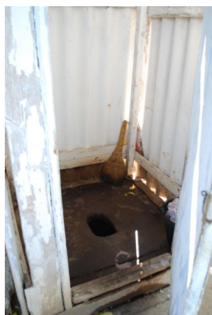
Figure 31 Pit latrine with a solid platform made out of concrete.
