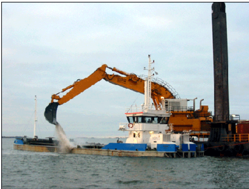
Figure 1 Mechanical dredging and placement of excavated sediments on a barge at Värmdö Garpen. ( www.sjofartsverket.se/pages/9266/allmant3.gif )
