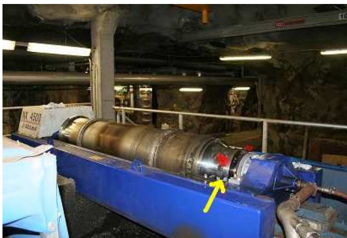
Figure 7. The disintegrating equipment partly mounted on centrifuge number 1 at Henriksdal WWTP. Photo: Stockholm Water.
