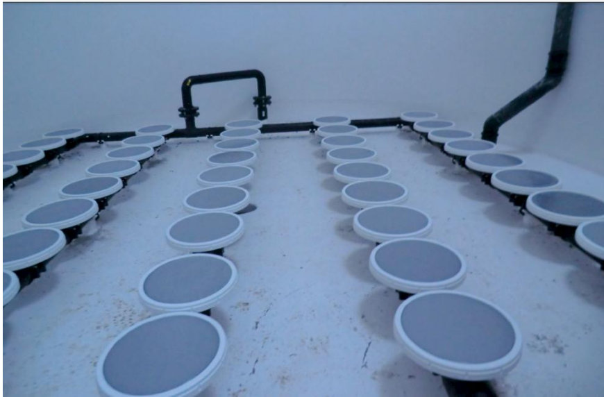
Figure 2 Blower plates on the bottom of the SBR at Kungsberget's WWTP.
